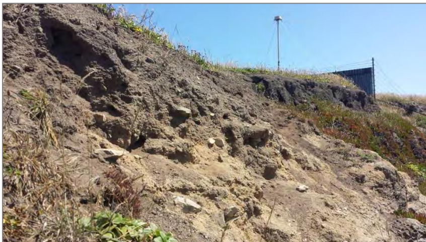
Figure 8. Bluff Edge Soil Profile. A top layer containing rubble and large angular rocks was evident in the top 3–4 feet of the soil profile.
